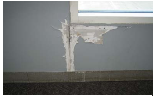
Damage at Holdroom Window Sills
