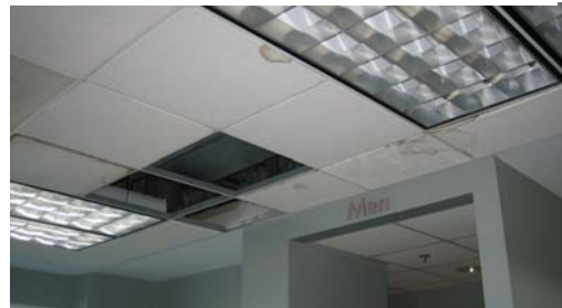
Water Damage at Holdroom Ceiling
